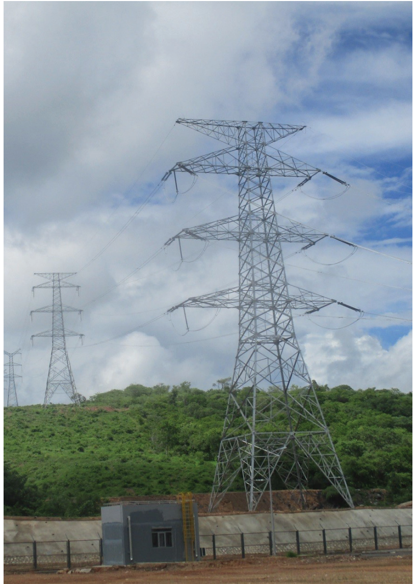
Powerlines along MCL's 40-km stretch to Muzuma sub-station.
