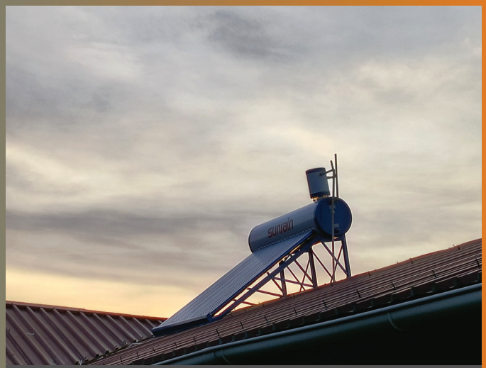
Solar Geysers Installed at Malaiti House
