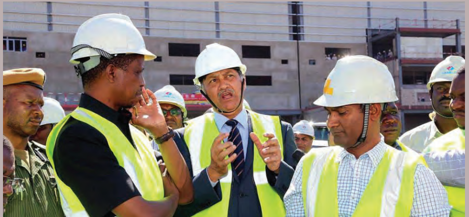
MCL Chief Executive Officer, Rear Admiral Venkat Shankar (Retd) explaining a point to Zambia's Republican President during the tour of the Thermal Power Plant (TPP) construction site on 16th September, 2015
