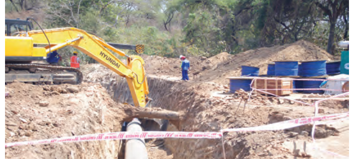
The Water Pumping system at Lake Kariba is nearing completion. The tank with the capacity to store 3 million litres of water has been pressure-tested and ready to operate.
