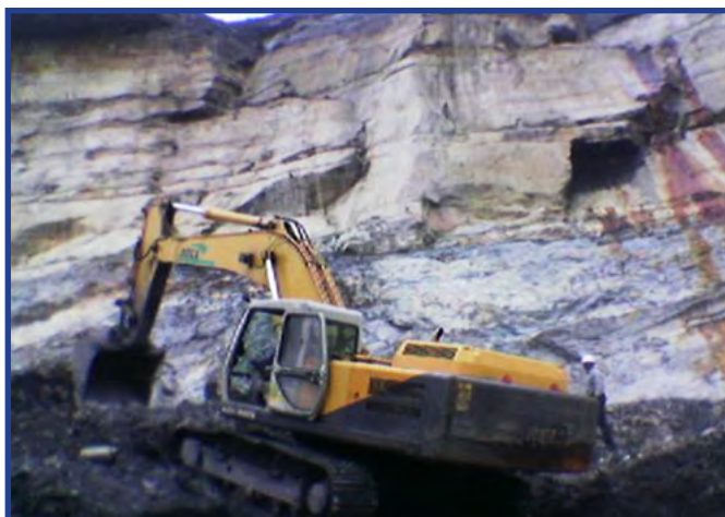
▪ Hired excavator mining coal just below and next to a very high wall at Izuma A
