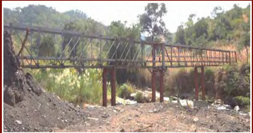
The Izuma foot bridge which has been constructed by MCL to promote the movement of people in some crocodile infested areas in Maamba.
