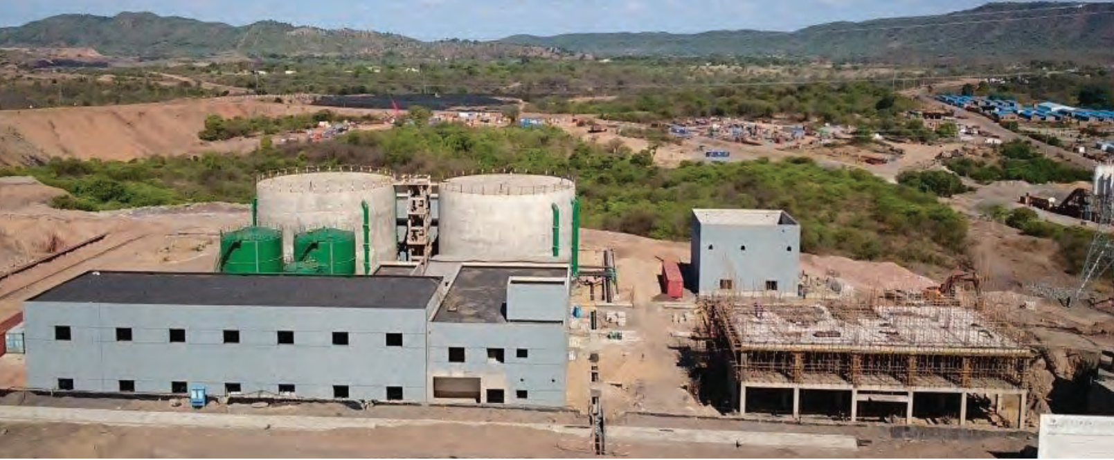
The (DM) Plant will be commissioned soon.
