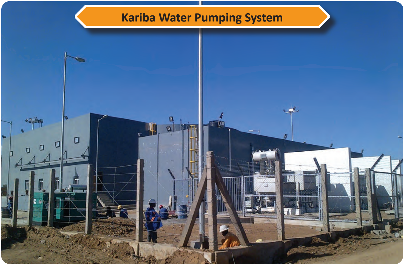
All the civil works at Kariba Lake Water Pumping System have been completed. Testing of high lift pumps, transformers, PLC and switchgear has been successfully completed. Pumping of water into the Raw Water Reservoir (RWR) has commenced.
