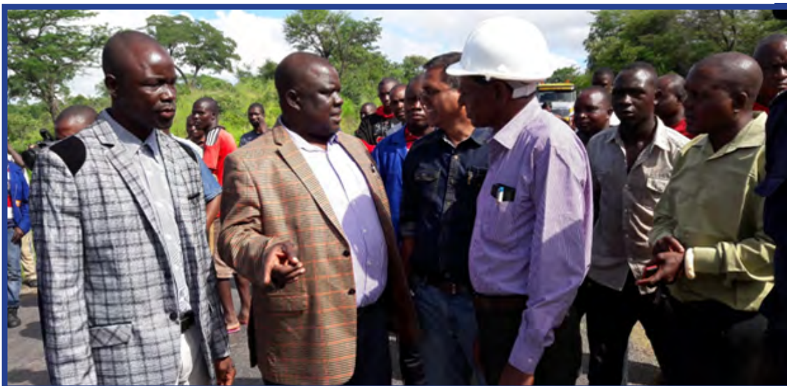
■ MCL Manager – Civil, Mr. Panthulu (in blue shirt), explains the extent of works to the Area MP, Hon. Sialubalo, (in brown jacket) after MCL deployed its equipment to repair the washed away Maamba – Batoka Road on 8th February, 2017.
