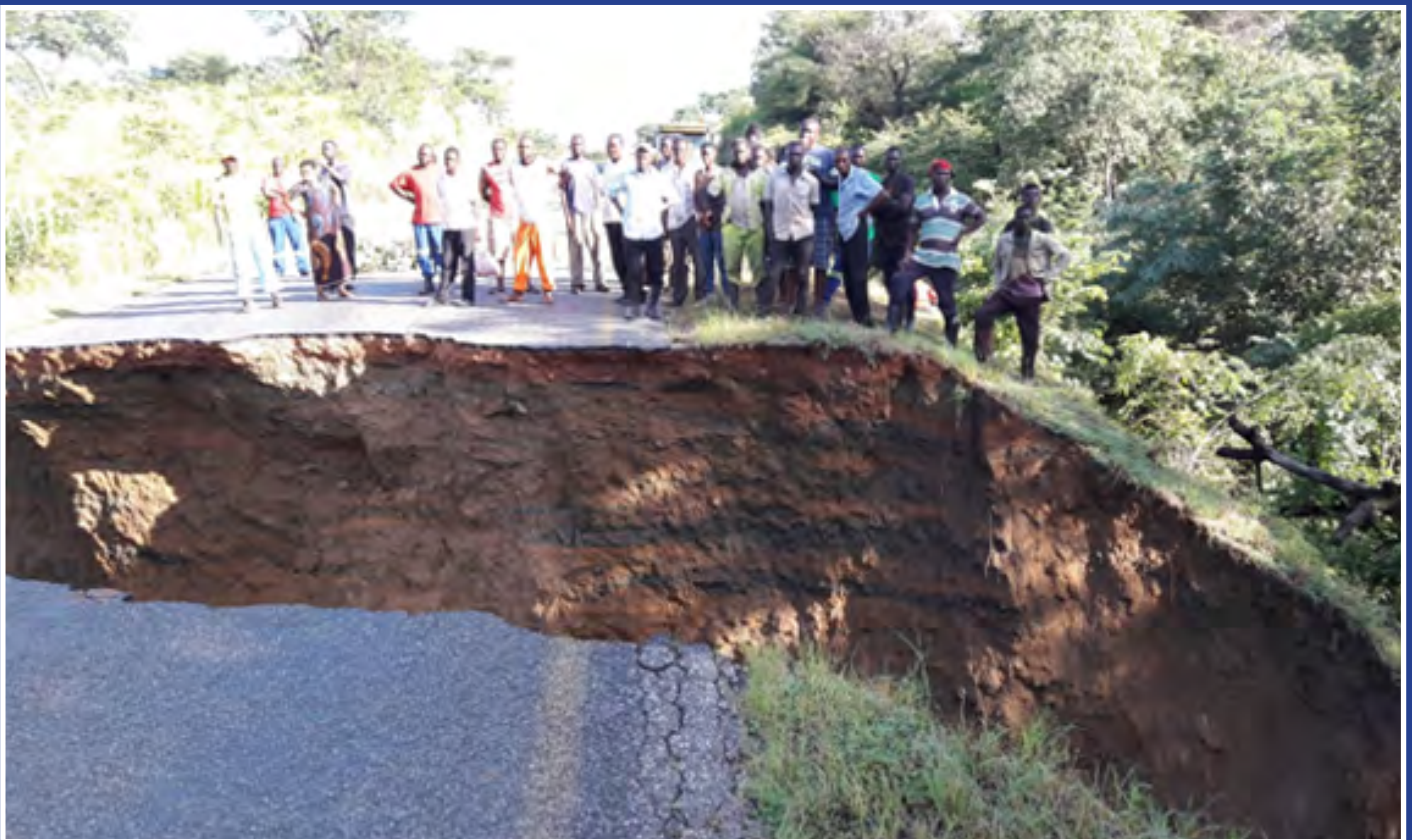
■ Washed away Maamba – Batoka Road
